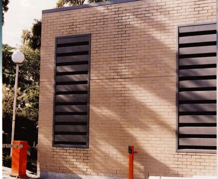
H-Line Louvres reducing plant-room break out noise
