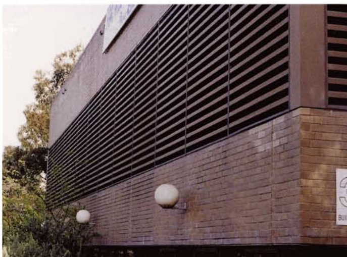
Multiple S-Line Louvre modules installed as a continuous wall
